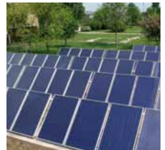
210 m 2 SOLAR THERMAL PLANT
