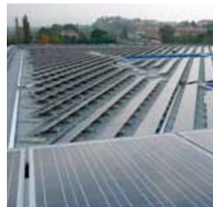
810 kWp PHOTOVOLTAIC PLANT
