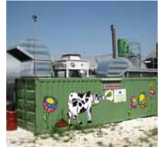
250 kWe BIOGAS PLANT
