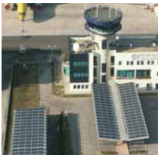
45,8 kW PHOTOVOLTAIC PLANT
