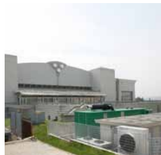
CHP VEGETABLE OIL-FUELLED 420 kWe PLANT
